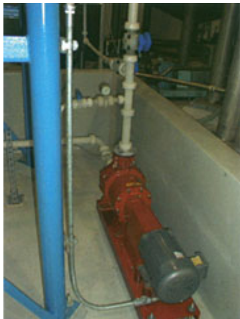
Figure 2: View of 12,500-gallon tank with Vanton CGM magnetically-coupled polypropylene pump for handling sodium hydroxide at 55 gpm against a 0 foot TDH.
