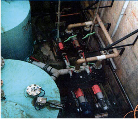
Overhead view of four thermoplastic centrifugal pumps handling discharges from the production area of a major silicon wafer facility in the U.K.. The process fluids include hydrochloric, nitric, sulfuric, hydrofluoric and phosphoric acids as well as hydrogen peroxide, caustic soda and other chemicals in unknown quantities.
