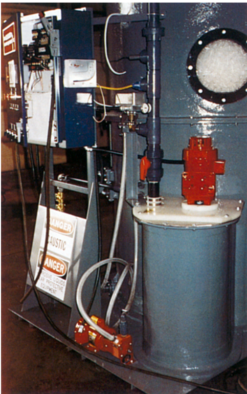
Gaylord H 2 SO 4 fume scrubbers use thermoplastic pumps and thermoset tanks to resist corrosives. Teflon rotary pump with Hypalon flexible liner transfers 50% NaOH to the fiberglass tank. The caustic in the tank is circulated by a polypropylene sump pump with cantilevered integral pump/motor shaft sleeved in plastic.
